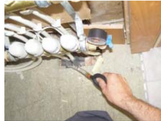
Underfloor Heating Manifolds
